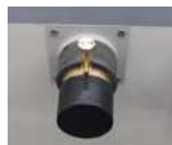
Header of cooling coil
