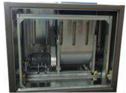
Figure 13. Electric Heater in AHU
