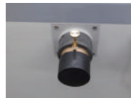
Cooling coil collector pipe
